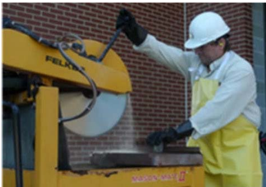
A worker cutting masonry block on a stationary masonry saw that continuously feeds water to the blade.
