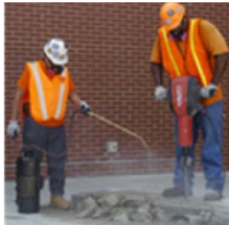
One worker applies water using a portable sprayer to suppress dust while the other jackhammers.
