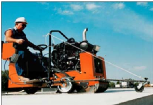
A construction worker cutting pavement using a drivable saw with an integrated water delivery system.
