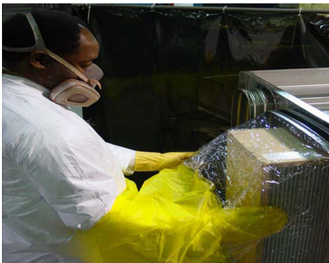
Figure 19. Removal of a dirty air filter from a ventilation unit into a plastic bag to minimize worker exposure to particles captured by the filter unit (Used with permission from Filtration Group Inc. [2012])
